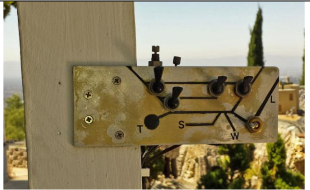
North End Switch Control
